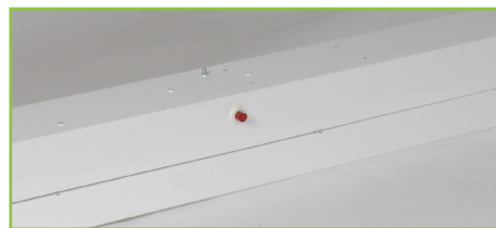
Battery Back Up (BB)
